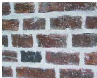
Above Poor brickwork with mortar joints that are messy, too wide and not tooled-in properly
