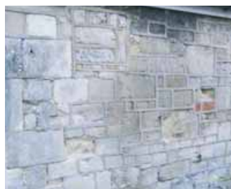
Above The use of ribbon pointing that stands proud of the stonework is inappropriate, uncharacteristic of the area and spoils an otherwise fine wall.
