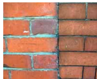
Above A crude junction between brickwork and mathematical tiles.
