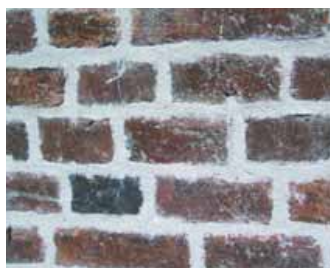
Above Poor brickwork with mortar joints that are messy, too wide and not tooled-in properly.
